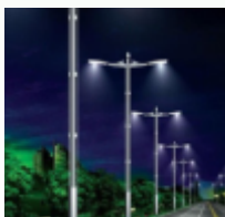
LED STREET LIGHTS
